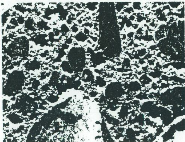
Plate 14. Excessive air content in concrete from highway pavement (air content = 30 percent). The pavement was rejected and removed. Magnification X 2.
