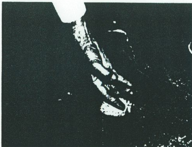
Plate 1. Scaling of a trowelled surface of a concrete floor in a furniture warehouse.
