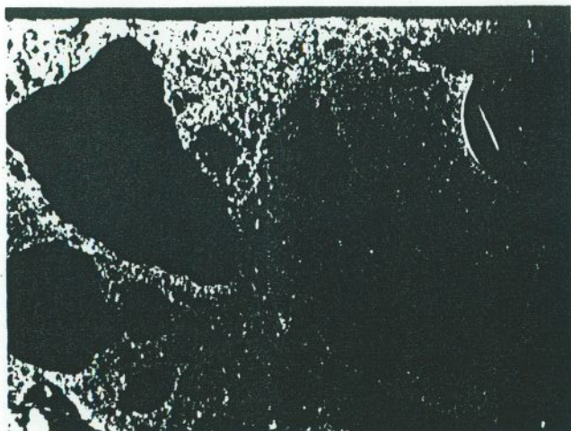
Plate 3. Extensive carbonation of the near-surface portion of base concrete of a floor placed in enclosures where unvented combustion heaters were employed. As a result of the weakened condition of the surface more than 30,000 sq. ft. of concrete topping became disbonded and required replacement. Magnification X 1.
