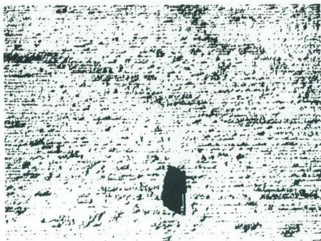
Plate 4. Sealing of finished surface of bridge deck concrete resulting from finishing and application of a membrane curing compound before completion of bleeding. Accumulation of bleeding water beneath the surface of the concrete resulted in immediate spalling of the topmost 1/16-1/8 inch.
