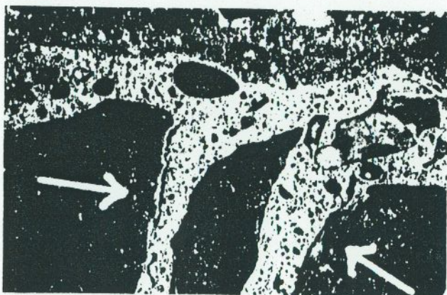
Plate 6. Cross-section of lining of a flume structure that displayed spalling of finished surfaces in limited areas. A weakly bonded layer of mortar at the top demonstrates poor finishing procedures whereby the surface was brought to grade by a mortar slurry that was not integrated with the underlying concrete. Fissures (arrows) demark bleeding channels; note that the channels are obliterated by the finishing operations. White masses of gypsum in the dolomite coarse aggregate had produced no deleterious effects. Magnification X 2.
