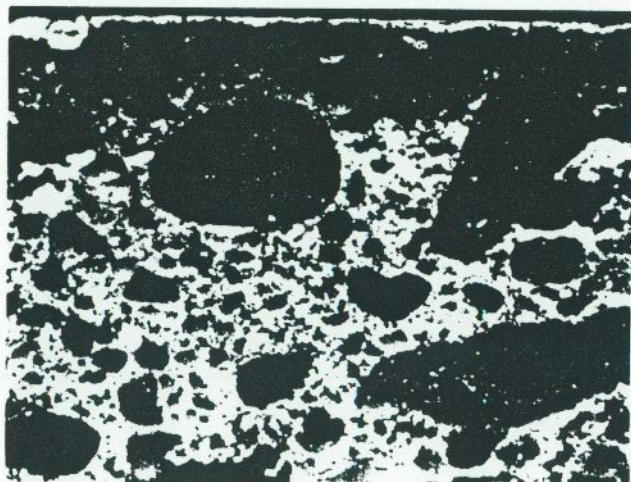
Plate 2. Cross-section of the concrete floor shown in Plate 1. Note the poorly bonded layer of sand-cement mortar applied to the surface and not integrated into the surface of the base concrete. The construction specifications called for a monolithic floor slab. Magnification X 9.
