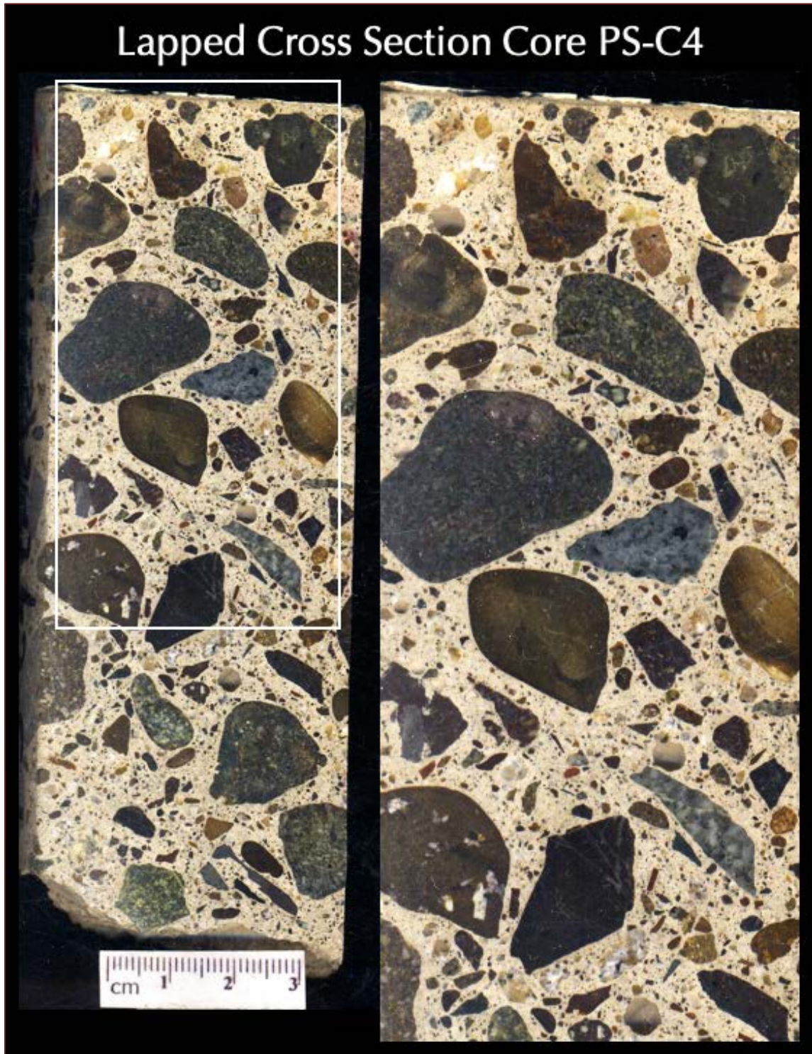
Figure 15: Lapped cross section of Core PS-C4 showing: (a) a thin paint coat at the top well-bonded to the underlying concrete having a nominal thickness of < 1 mm; (b) the main concrete body containing crushed volcanic and volcanoclastic gravel coarse aggregate where aggregate particles are subrounded to subangular, dense, variably colored, well-graded, and well-distributed, natural siliceous sand and finer fractions of volcanic rocks and minerals in fine aggregate, all dispersed in a Portland cement paste; and, (c) the overall sound (visually crack-free), dense, well-consolidated nature of the concrete in the body. The boxed area at left is enlarged at right.
