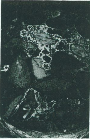
FIG. 24. Polished surface of concrete which is coated with gel which appears white. The gel issues onto the polished surface through fine cracks which occur on the aggregate surfaces. To the bottom and right of the photograph white gel can be seen along the aggregate surfaces in the fine cracks. Width of photograph = 60 mm.
