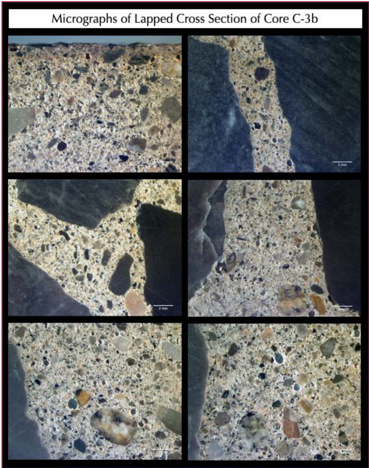
Figure 26: Micrographs of lapped cross section of Core C-3b showing: (a) the overall non-air-entrained nature of concrete having a few discrete, spherical and near-spherical entrapped air bubbles, and (b) overall porous but well-consolidated nature of concrete.
