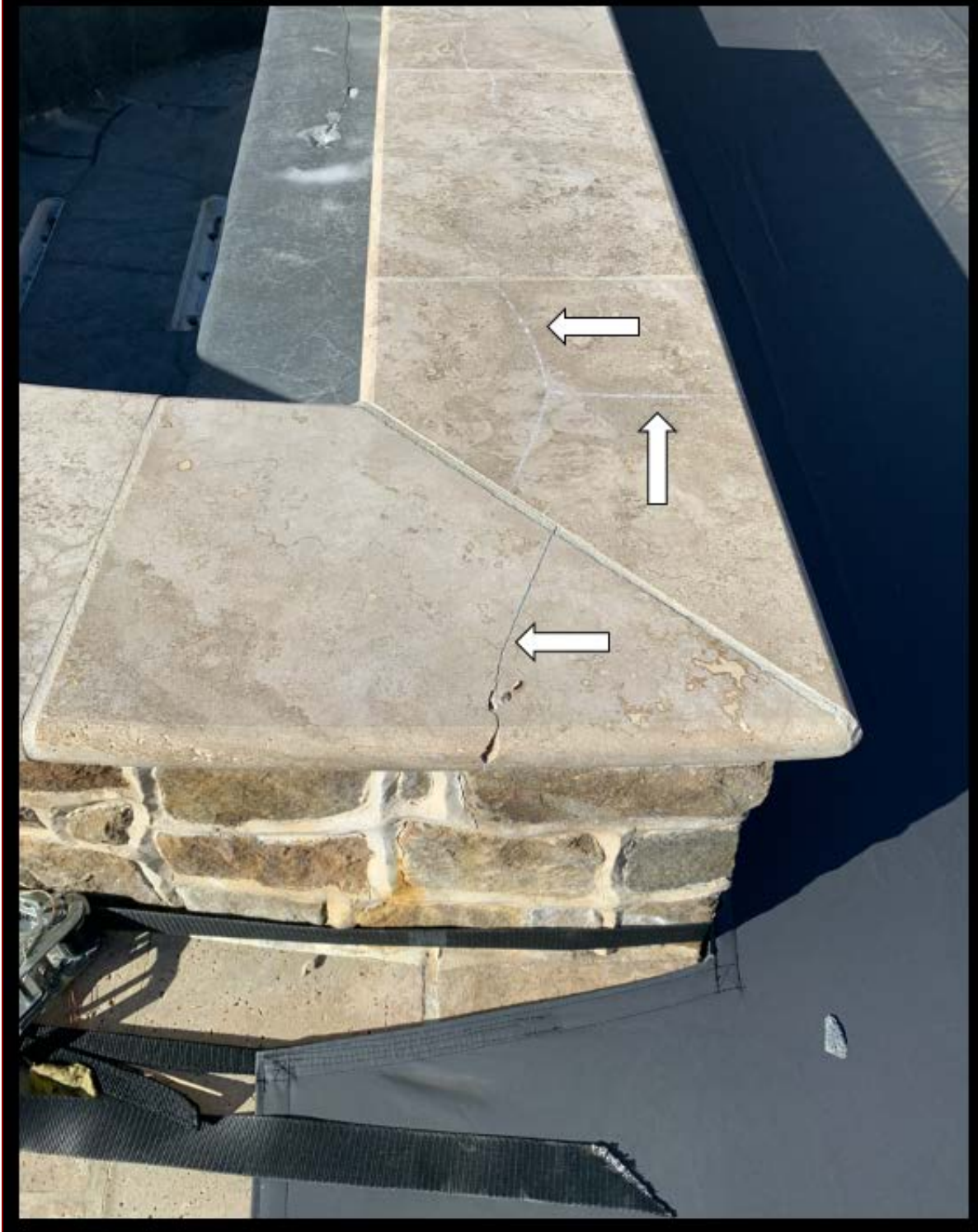
Figure 3: Enlarged view of some fine, visible cracks on the limestone tiles around the spa.
