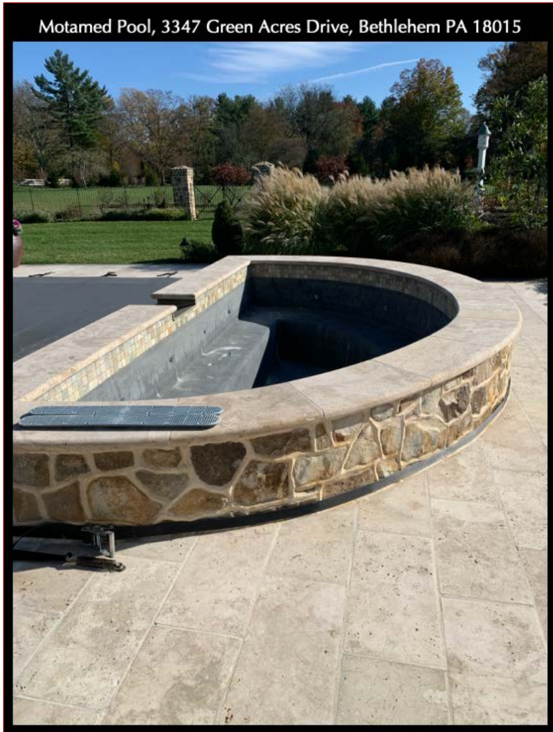
Figure 1: Field photo of the spa area of swimming pool showing limestone tiles on pool deck and masonry wall around the spa. The present investigation addresses extensive cracking in the dark gray pool plaster within the spa area.
