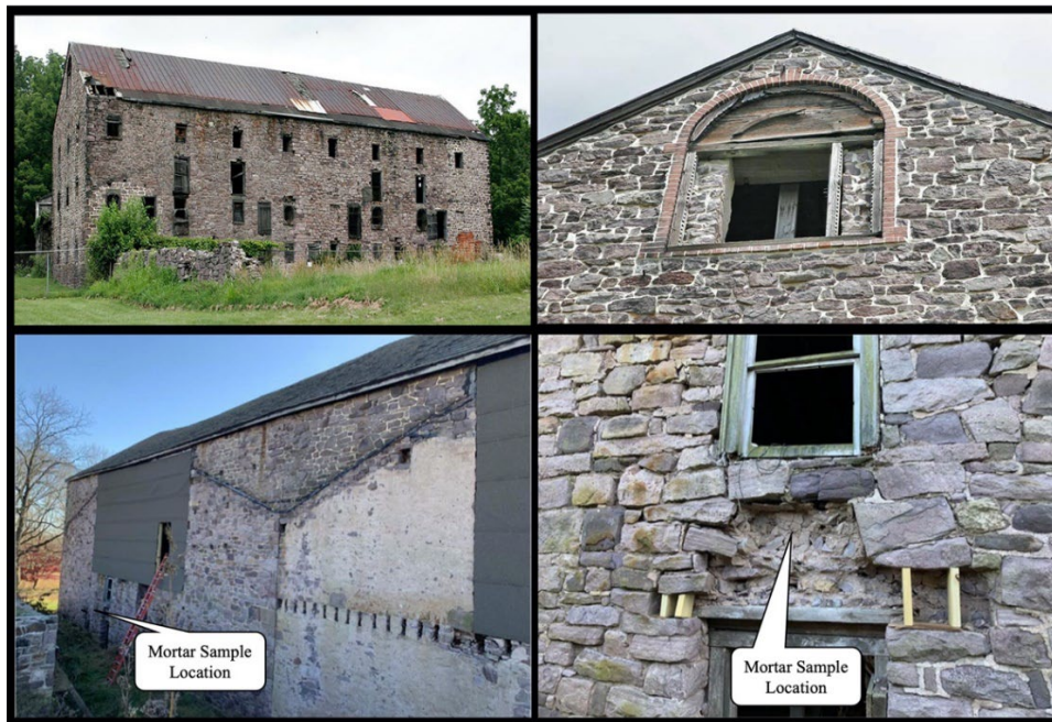
Figure 1 - Field Photos of Wetherill Barn at the Valley Forge National Historic Park Showing Location of Bedding Mortar Sample
