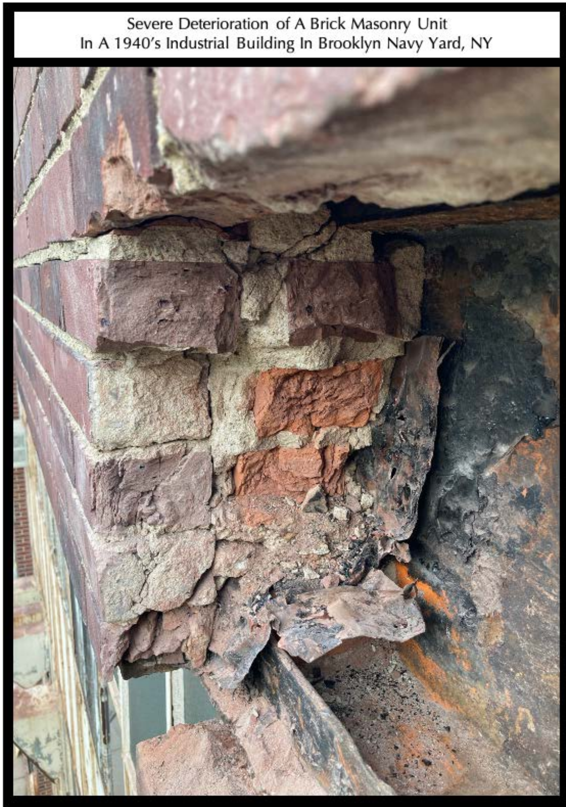
Figure 3: Another field photo of masonry wall showing different color tones of brick masonry units and medium gray jointing mortars.
