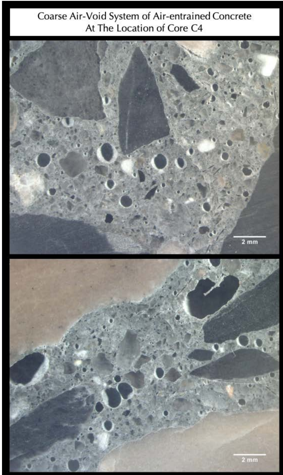
Figure 30: Micrographs of lapped cross section of Core C4 showing the marginally air-entrained nature of concrete having mostly coarse air voids at moderate amounts, as opposed to excessive air-entrainment of many very fine air voids as seen in Core C1.
