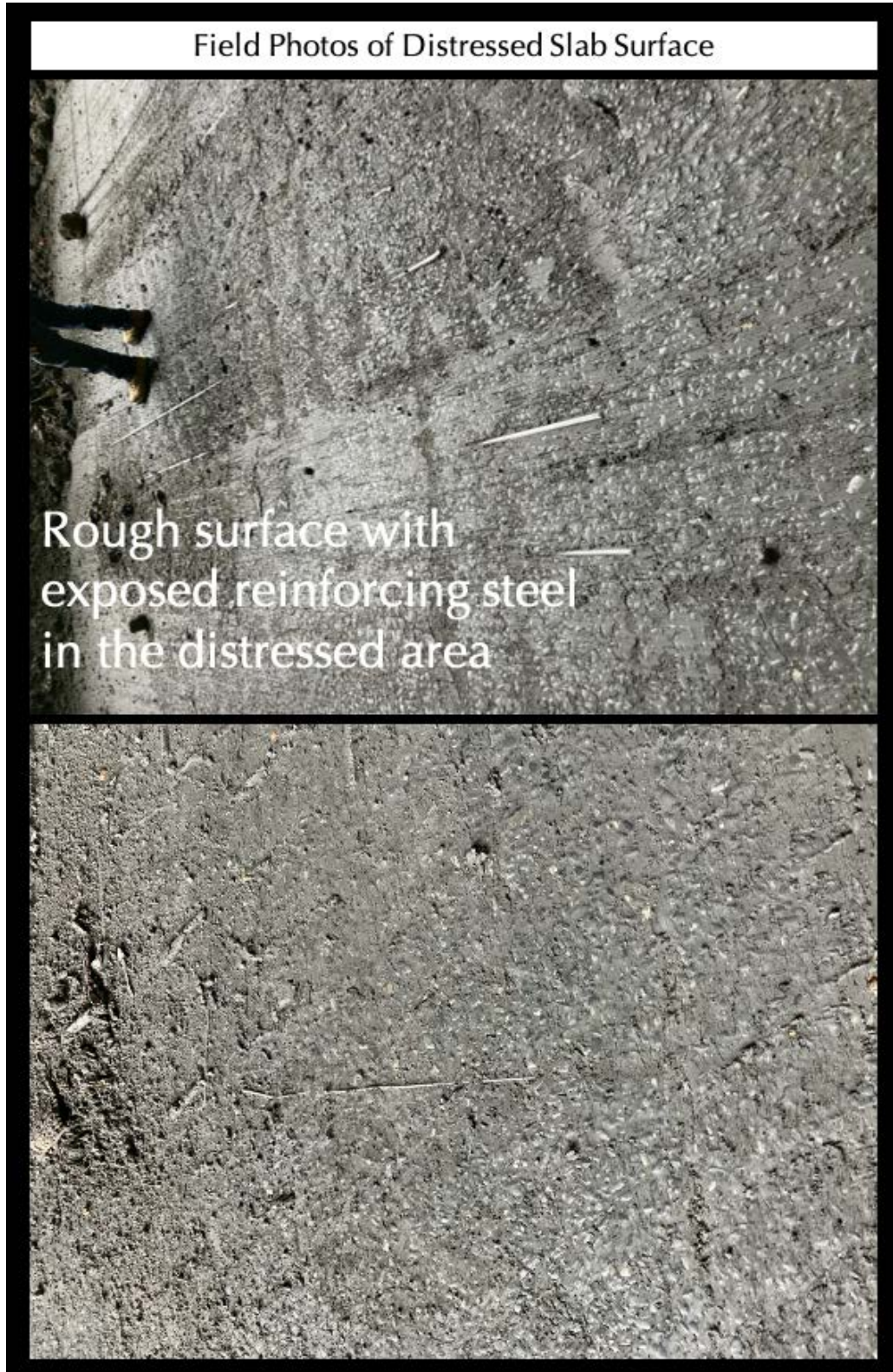
Figure 3: Field photo of the distressed concrete slab surface showing rough surface with exposed reinforcing steel at the surface where the original trowel-finished surface has, reportedly, delaminated.
