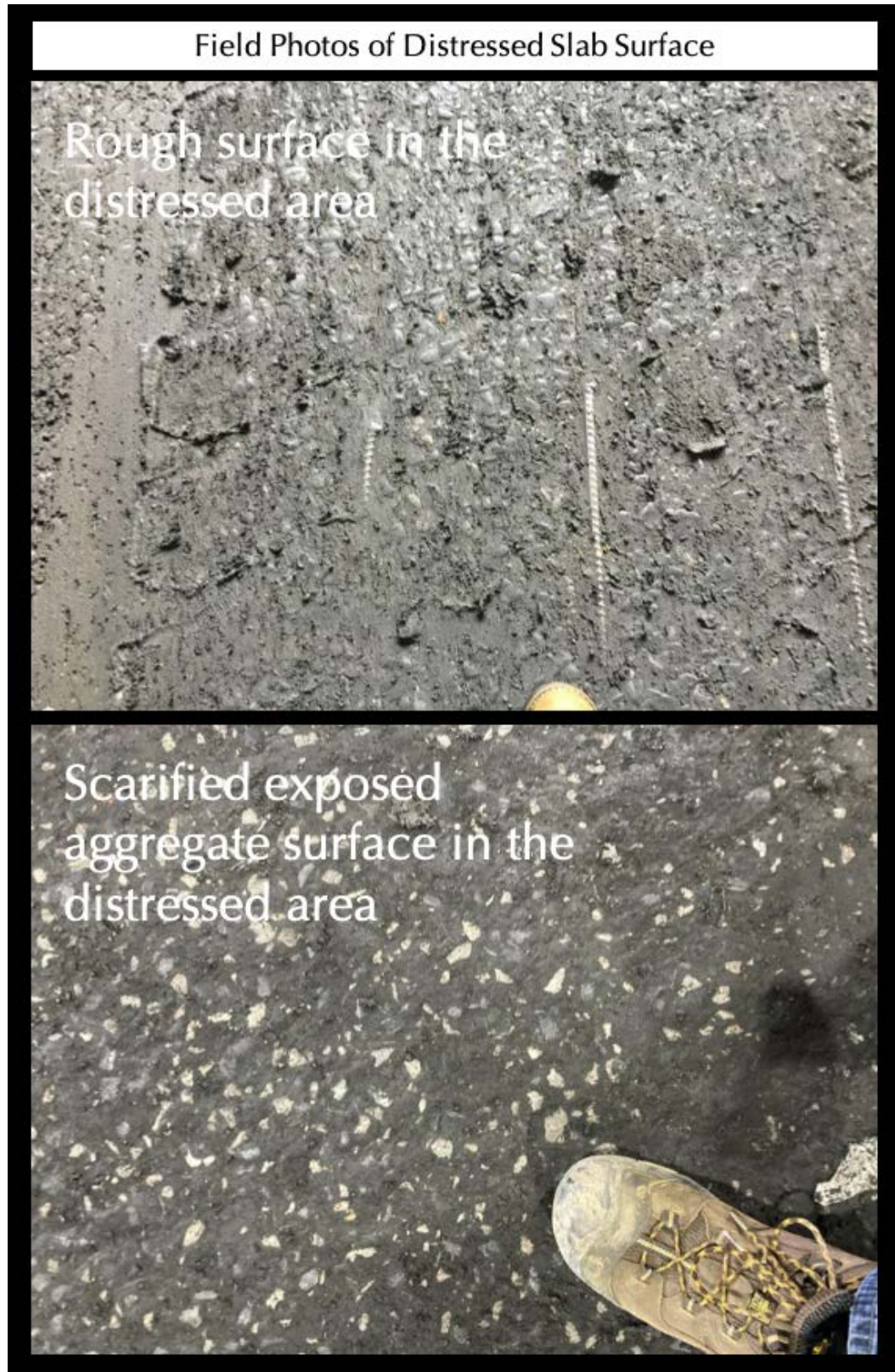
Figure 2: Field photos of rough distressed area in the top and scarified surface in the bottom photos that were subjected to delamination from loss of the original densified trowel-finished surface.
