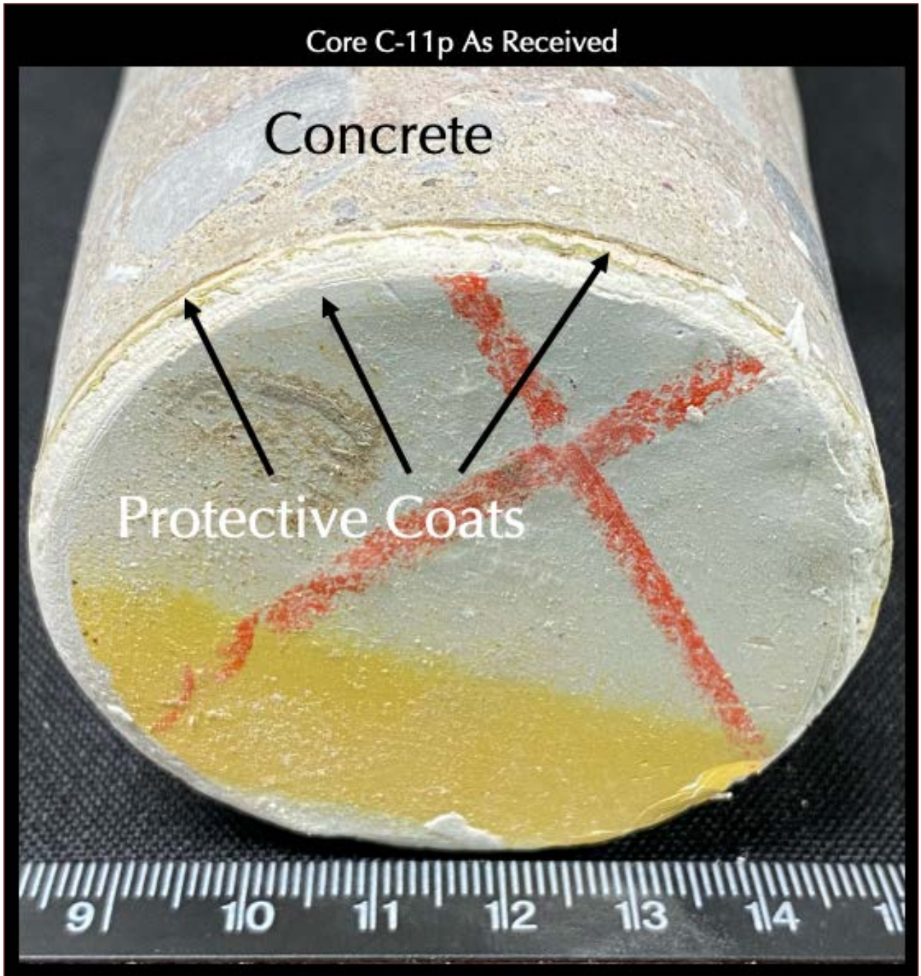
Figure 2: Core C-11p from Column 21, Ground Level, as received showing an off-white protective paint coat and a few more layers of a protective coating system, which is well-bonded to the underlying concrete body.
