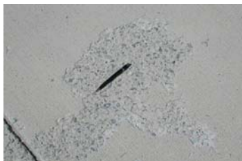
Fig 1: Scaling of Concrete Sidewalk
