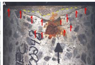
Spalling due to corrosion of reinforcing steel in concrete
