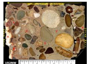
Concrete exposed to high temperature in a chimney
